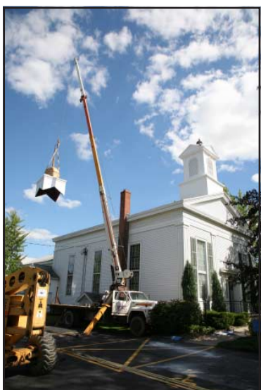
The dome begins its journey to the top after being picked up from the ground.
