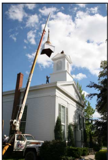
The trip is almost over as the dome approaches the cupola, under the direction of a worker on the roof.
