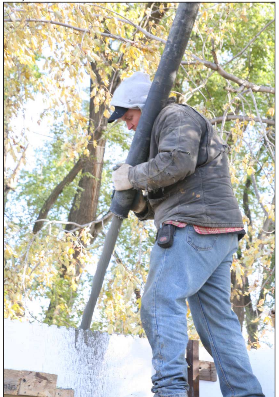
Brent Bricklin , president of O'Bricklin Mason Contractors, feeds the slurry into the top of the forms. It took about one hour to finish the walls, using 22 yards of high slump concrete.
