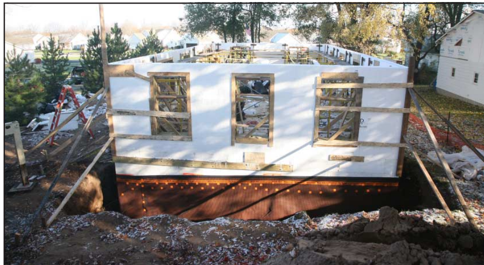
The house on Lyell Avenue in Spencerport before the concrete was poured. All the window and door openings are braced to withstand the pressure of the concrete.
