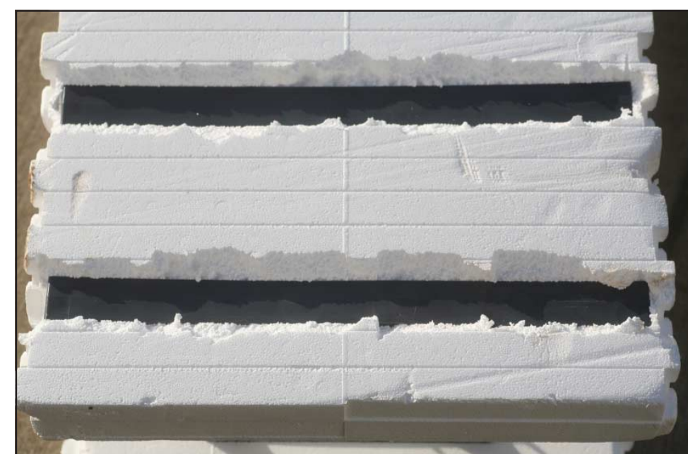
Two sections of an Insulated Concrete Form were broken out to reveal the plastic pieces imbedded behind about 1/2 inch of polystyrene. These two inch plastic panels are used as anchor points which allow attaching siding to the outside wall of the form and sheetrock to the inside wall of the form. Electrical and plumbing lines are routed out of the inside wall before the sheetrock is attached.
