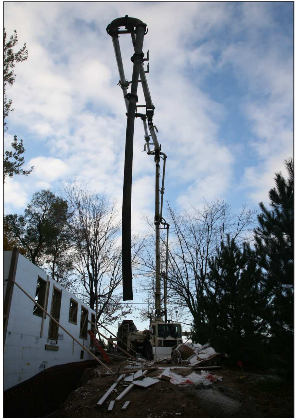
The feed system utilizes a concrete pump truck and a boom with articulated control arms from which metal tubes are suspended, ending in a ten-foot rubber tube which delivers the concrete slurry to the forms. The slurry is held in a tank on the back of the truck which is fed from concrete delivery trucks.
