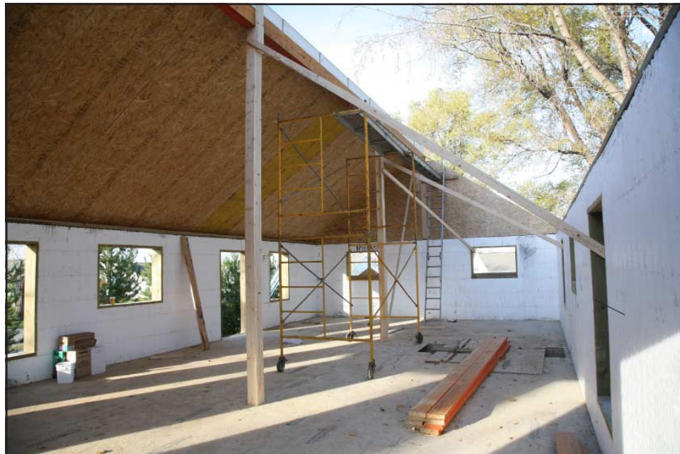
This interior view shows the support poles holding the ridge beam with half a roof yet to be fitted with panels.
