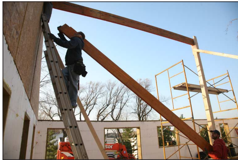
Brian Cansdale inches the second ridge beam up to the support post. The ridge beam consists of three side-by-side OSB's (Oriented Strand Boards), each one a 15 layer laminated board which is denser than plywood.
